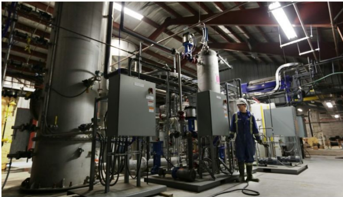
CE's pilot pellet reactor and associated equipment. (Carbon Engineering Ltd.)
