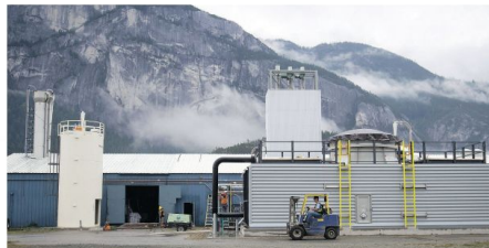
A worker drives a forklift at Carbon Engineering's first direct air capture plant in Squamish, B.C. The plant extracts carbon dioxide directly from atmospheric air in a closed-loop industrial process and turns it into gas suitable for use in a variety of applications.
